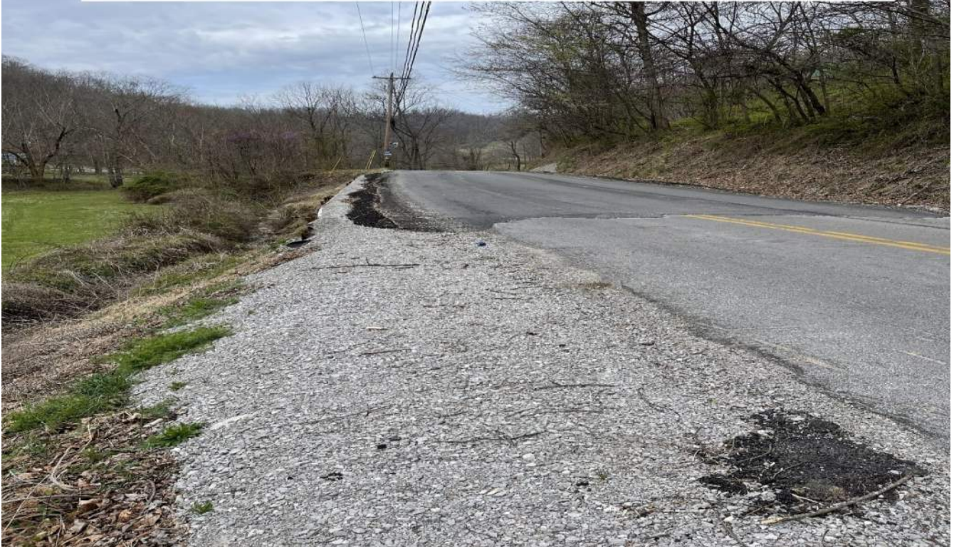
Previously Repaired Embankment Failure (Approximately MP 2.9)
